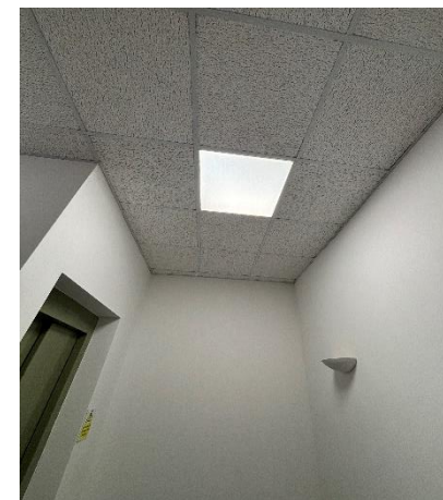
7. Lift ground floor
