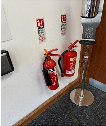
17. Fire extinguisher example
