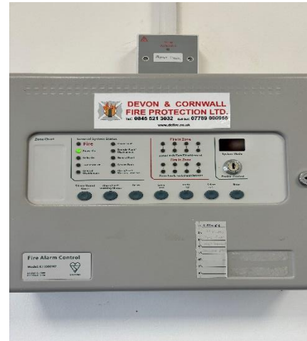
15. Fire alarm control panel
