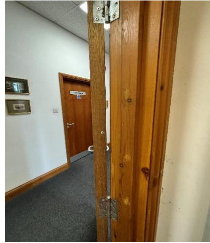
11. Certified fire door
