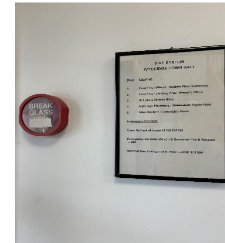
16. Incorrect fire zone plan
