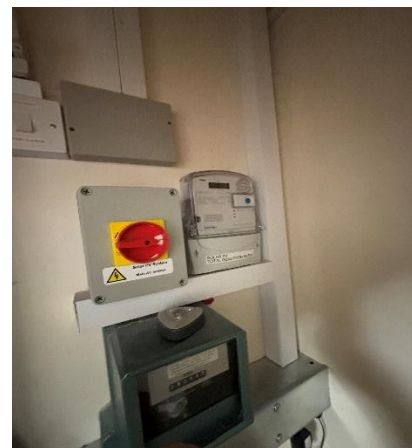
30. Solar shut down switch
