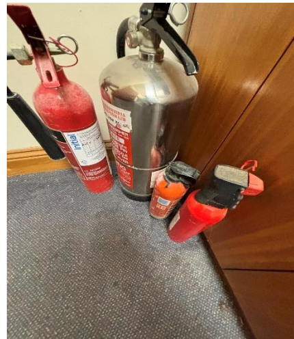
18. Fire extinguisher to remove
