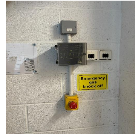
36. Emergency gas shut off (manual)
