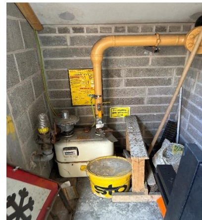
31. Gas intake room
