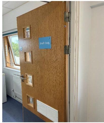
10. Fire door with vent
