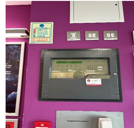
4. Fire alarm control panel
