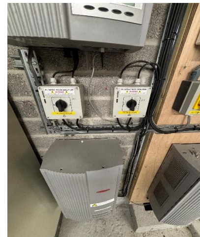
15. Solar PV inverters
