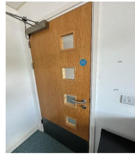
12. Fire door excessive gaps
