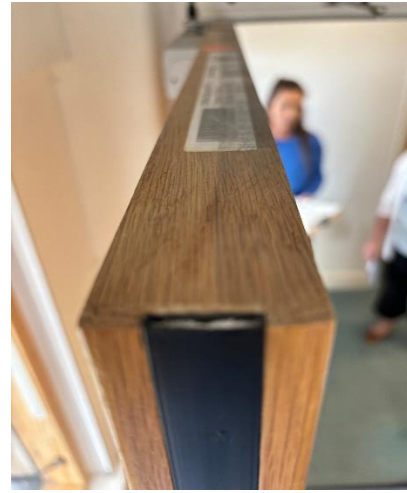
11. Certified fire door
