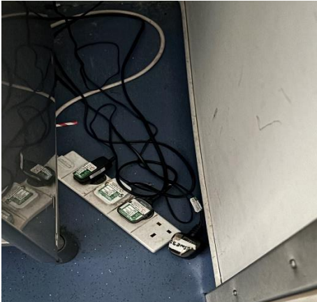
45. Extension lead usage
